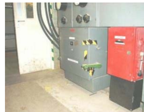
Fig 1 The LV breaker
